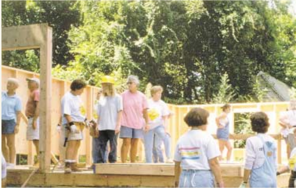
A new Habitat For Humanity home takes shape on Miner Street in Groton in this 2001 photo. EB employees have contributed their time and energy to this and other Habitat projects in the past few years, and they are now raising funds for a Habitat build in Waterford.
