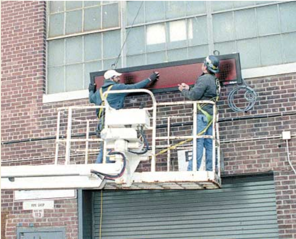
One of four new LED reader-boards is installed outside the Wet Dock Pipe Shop in Groton this month as part of the company's new electronic communications system to be known as EBTV.
